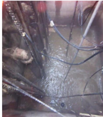
Figure 2. The lift station has remained clean since the installation of the PHI mixer in November of 2016.
