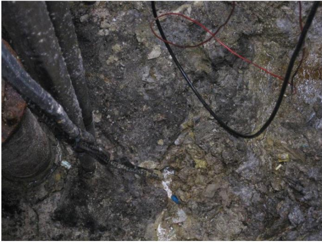
Figure 1. Excessive grease and rag buildup in wet well
